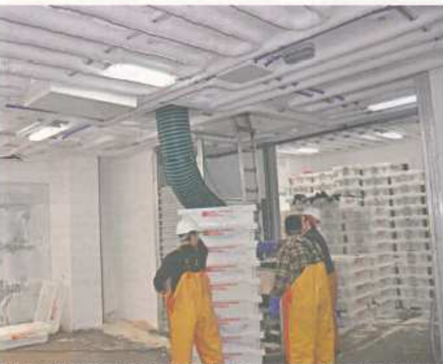
E. & R. Refrigeration installed the chilling, flake and slurry ice systems in the fishroom of Endeavour IV .
