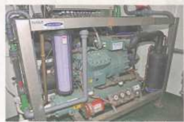
The machinery for the slurry ice system aboard Endeavour IV . Up to 15 tonnes of slurry ice at 10°C is produced every 24 hours by an S8 system supplied by Slurry Ice Systems Ltd. (SIS) of Scotland.
